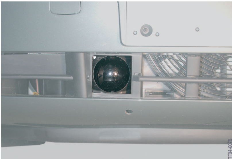
1 - ACC sensor installation location
